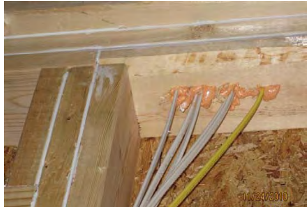
air infiltration caulking
