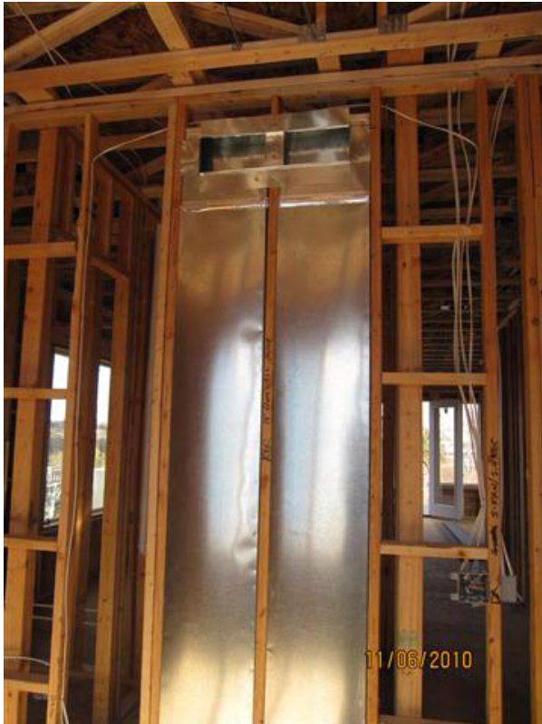
vertical HVAC ducting
