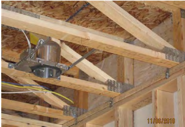
truss hold down straps
