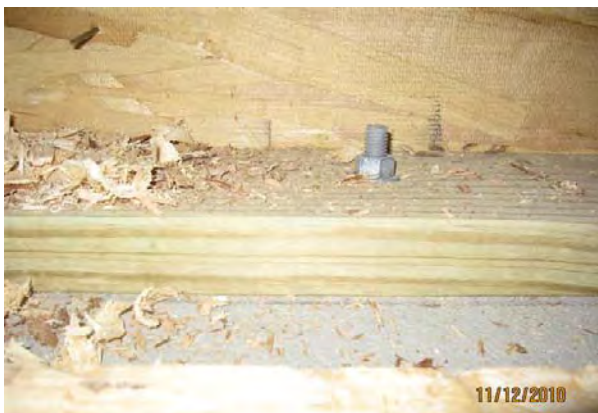
wood sill plate sealer separation
