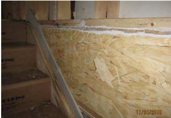
air infiltration caulking
