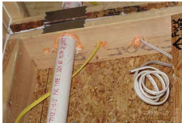
air infiltration caulking
