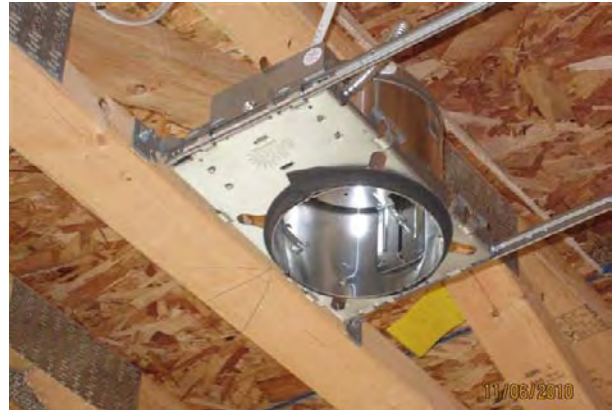
light fixture gaskets @ insulated roof
