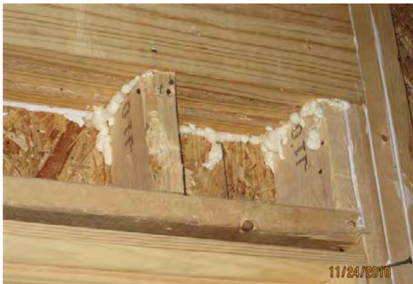
air infiltration caulking
