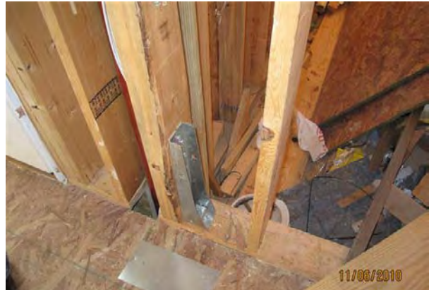
interior hold down brackets
