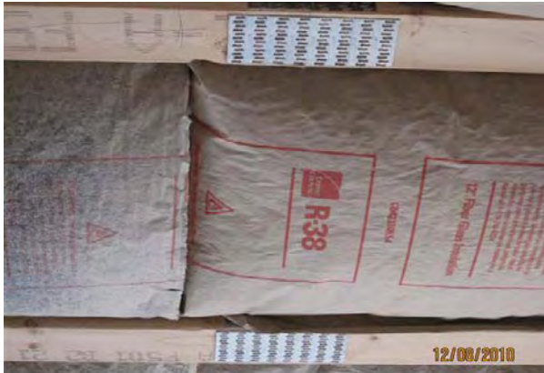
R-38 roof insulation
