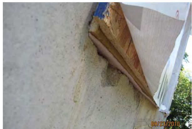
wood sill plate sealer separation
