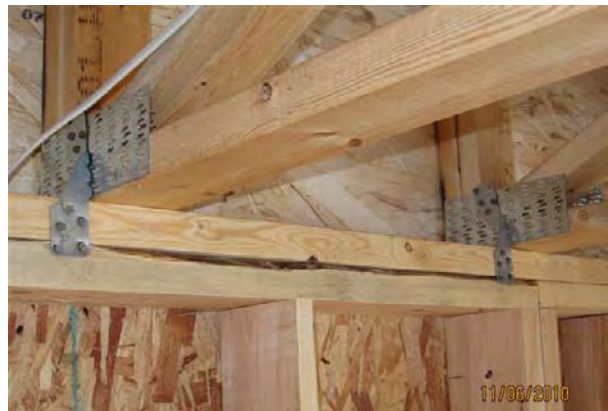
truss hold down straps
