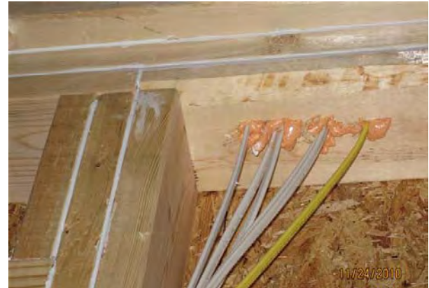
air infiltration caulking
