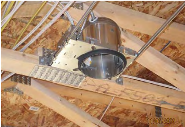
light fixture gaskets @ insulated roof
