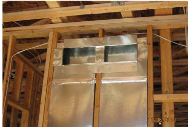
vertical HVAC ducting
