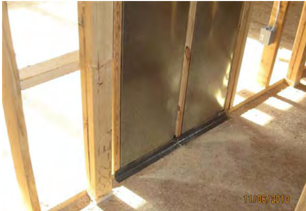
vertical HVAC ducting
