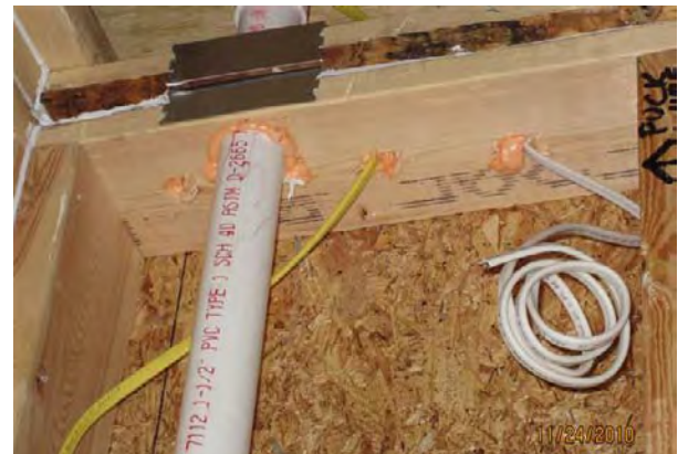
air infiltration caulking
