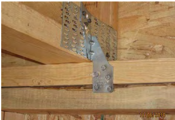
truss hold down straps
